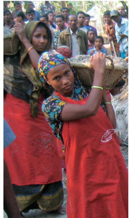
Bangladeshi women are building a road with support from Danida. Small as well as big projects are sought adapted to climate change. Photo: Jan Møller Hansen, Danida
